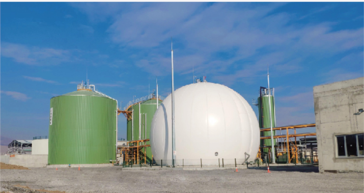
Processing capacity: Kitchen waste 150t/d
