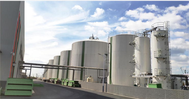
Processing capacity: Kitchen waste 400t/d
