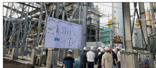
9MW Biomass Gasification Project (Vietnam)
